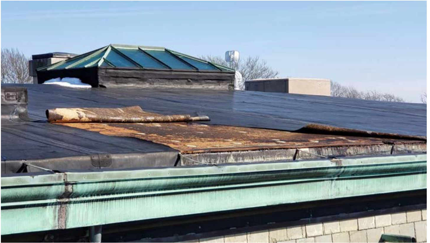
The Elms roof is showing its age, as are the roofs at Rosecliff and Marble House.
