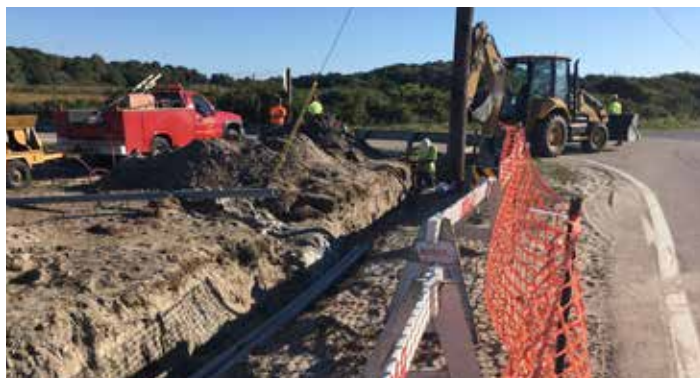
Above: Burying power lines along Sachuest Point Road will help to restore the historic viewscape.
