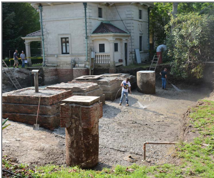
The roof of the underground boiler room at The Breakers is visible for the first time in a century, in preparation for waterproofing. Photo: Andrea Carneiro
