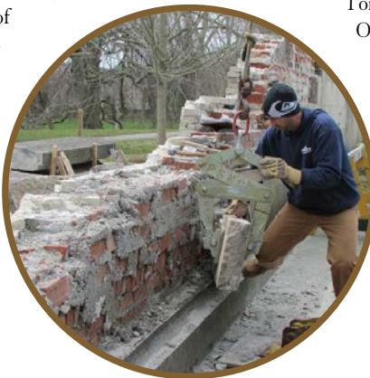
Rob Raffa of the Properties Department works on removing blocks from the north wall of The Elms, which was rebuilt. Photo by Andrea Carneiro
