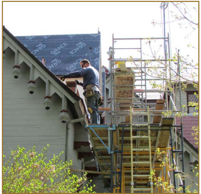
Work continues on the exterior restoration of Kingscote. Photo by Andrea Carneiro
