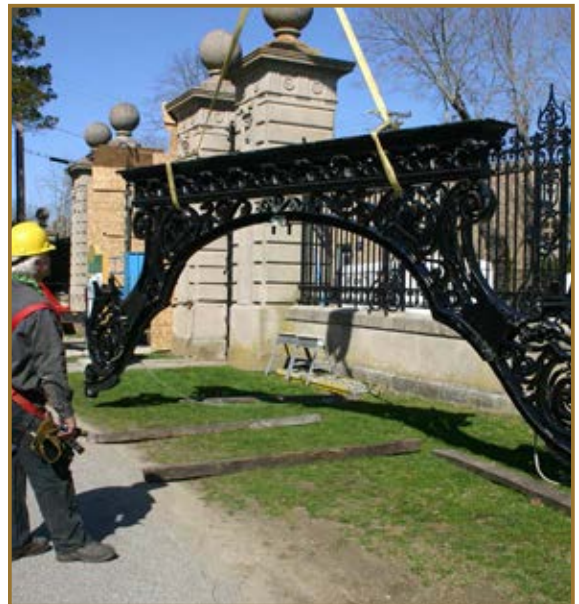
Donald Buschgans of Lodi Welding directs a crane as it lifts the crown of the north gate back into place at The Breakers after restoration. Photo by Andrea Carneiro
